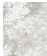
CRACKED STONE WALL P-VL880
